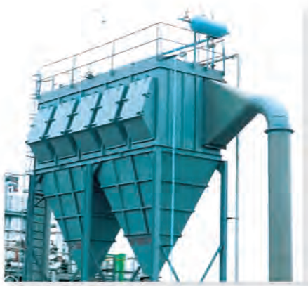
用于岐星水泥厂煤磨收尘的 高浓度、防爆型袋收尘器FGM96-5 ( M ) High Concentration, Explosion Proof Bag Dust Collector FGM96-5(M) used on kiln inlet in Qixing Cement Plant.
