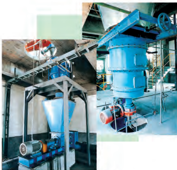
内蒙古华立水泥有限公司5000t/d生产线 回转窑、分解炉喂煤系统 Coal feed system for both the rotary kiln and pre-calciner of a 5000 t/d production line at Huali Cement Co.,Ltd Inner Mongolia
