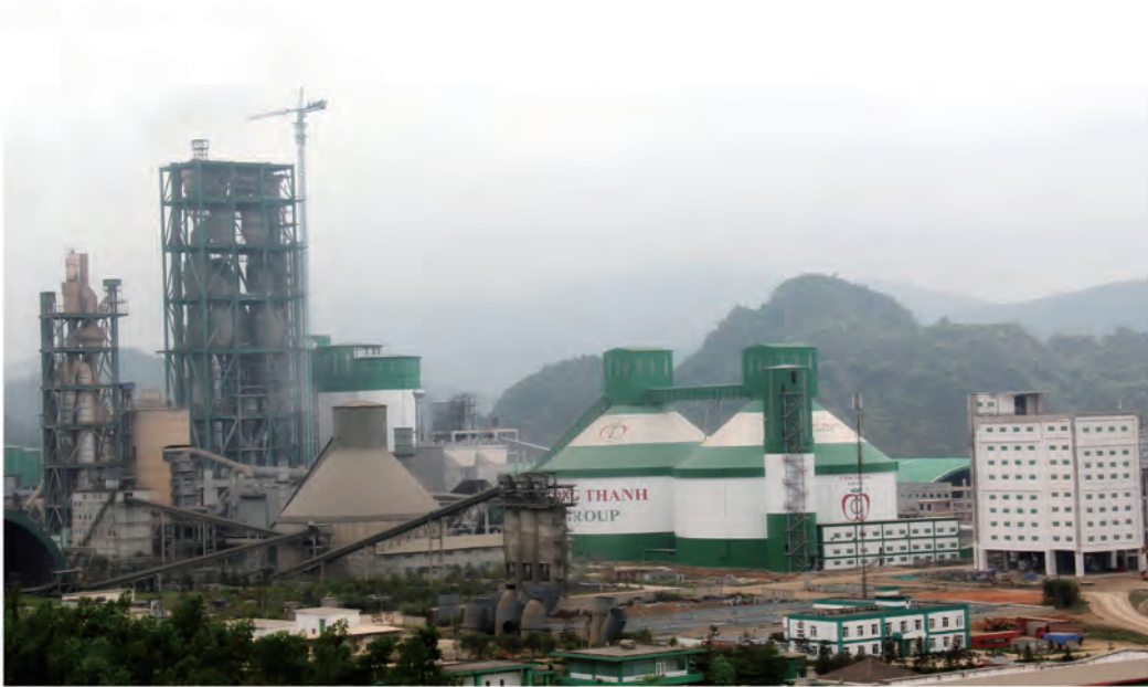
越南公清水泥有限公司12000t/d熟料生产线（在建中） 12000t/d Clinker Production Line at Cong Thanh Cement Joint Stock Company Vietnam (in construction)
