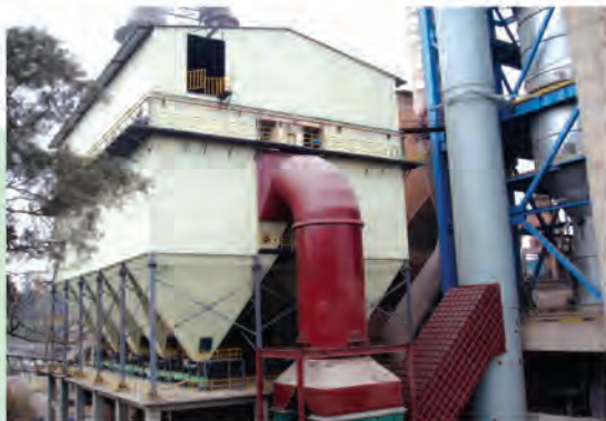
广州珠江水泥厂5000t/d熟料生产线窑尾袋收尘 Bag filter used on kiln inlet at Guangzhou Zhujiang Cement Plant 5000t/d clinker production line
